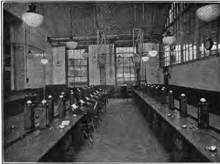
FIG. 2.—NEWCASTLE PHONOGRAM SWITCHROOM AFTER MODIFICATION FOR USE WITH AUTOMATIC DISTRIBUTION EQUIPMENT.
