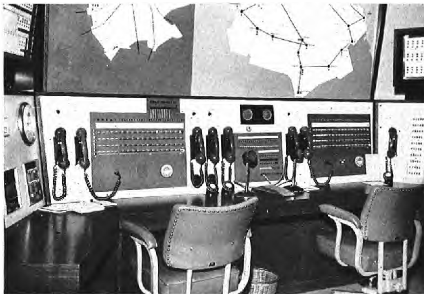
The priority-signalling panel is fitted above the left-hand switchboard; the miscellaneous-control panel is in the centre.
