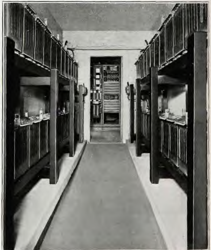
The Battery Room
