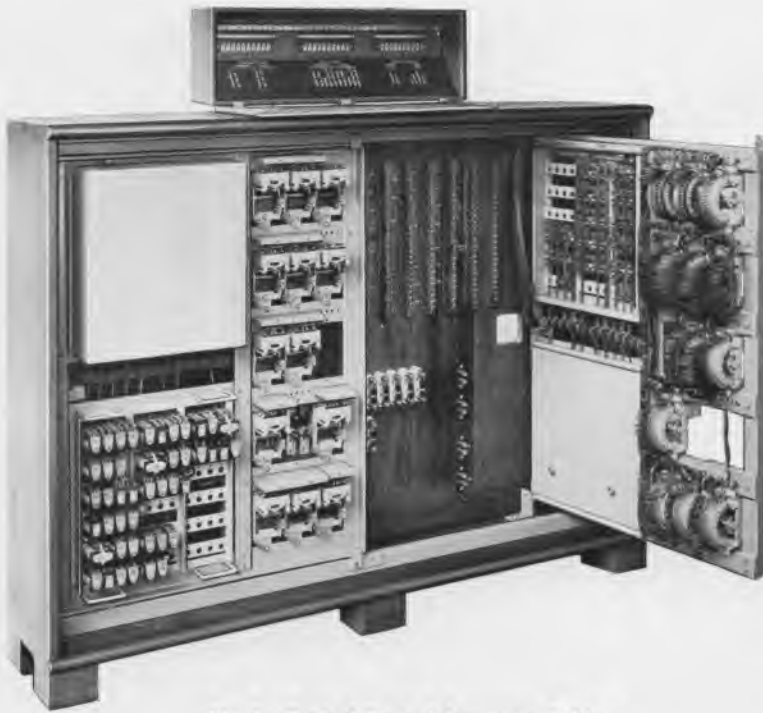
Fig. 8.—Typical Control Apparatus Cabinet.
