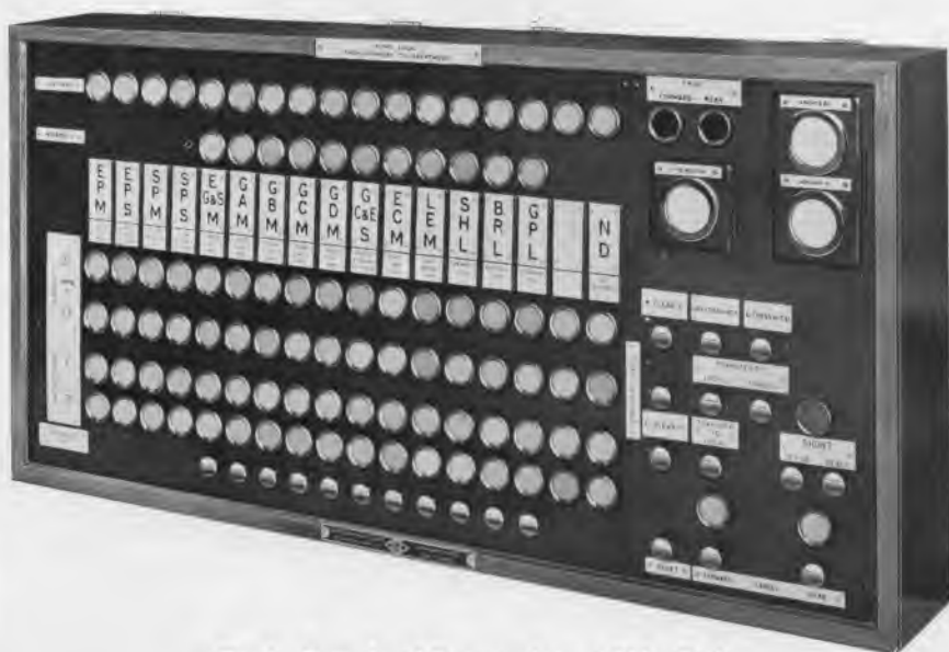
Fig. 4.—Down Local Retransmitter at Gidea Park.
