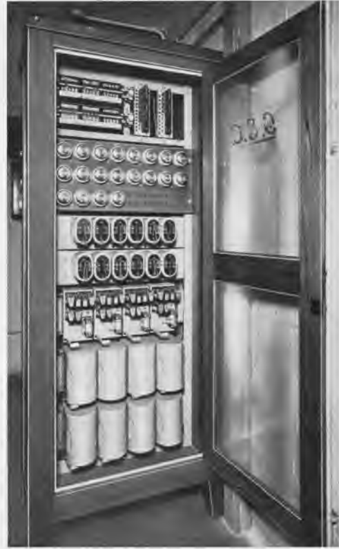
Fig. 7.—Apparatus cabinet at Newcastle.
