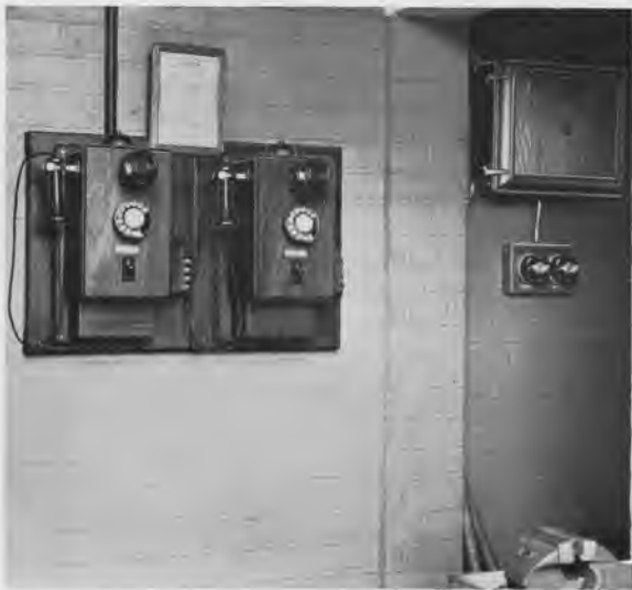
Fig. 4.—Selective ringing telephones at Woking.
