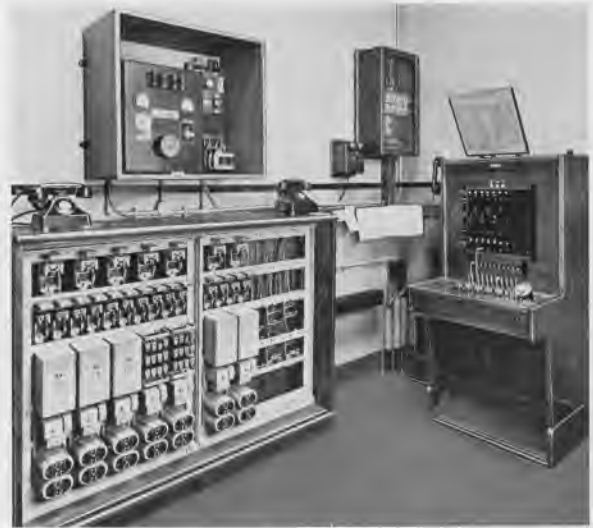
Fig. 7.—Switchboard and automatic apparatus at Woking.
