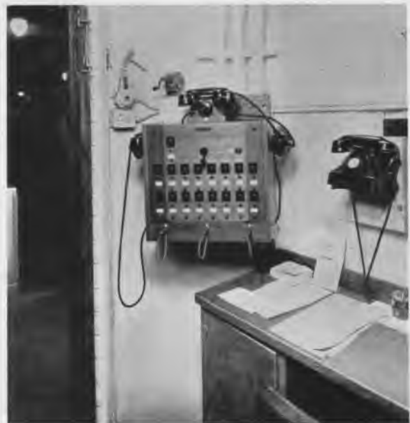
Fig. 2. —Kitchen clerks' cabinet, at which calls from stewards for room service are answered.
