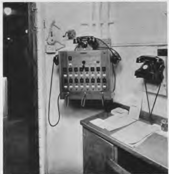
Fig. 2.—Kitchen clerks' cabinet, at which calls from stewards for room service are answered.
