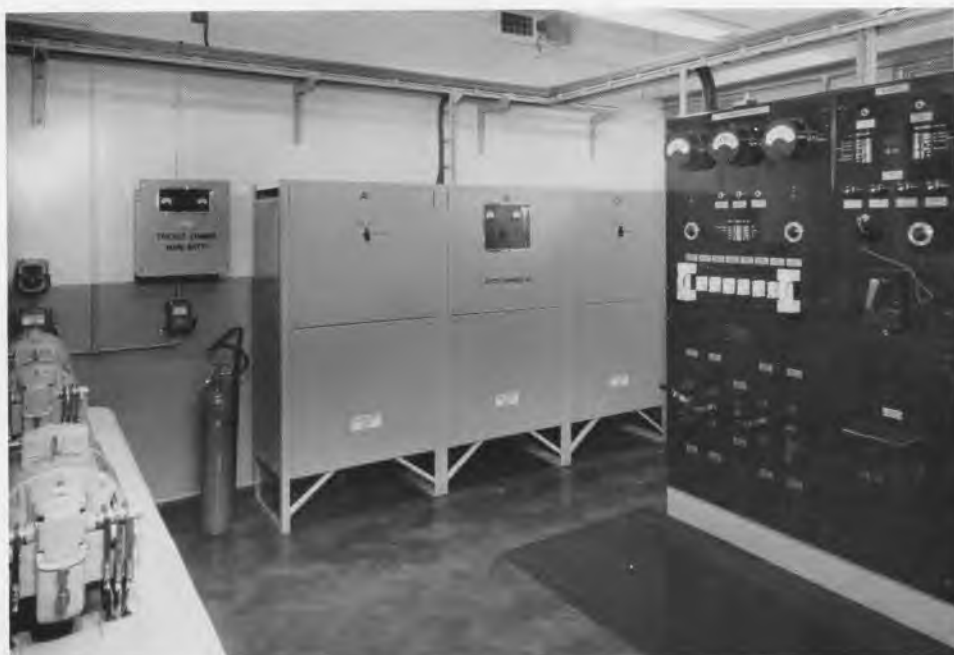
Fig. 1.—Power room with ringing machines on the left, battery charging equipment and main power switchboard.
