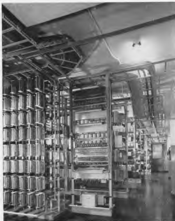
Fig. 3.—General view of the exchange showing the equipment racks and cabling.
