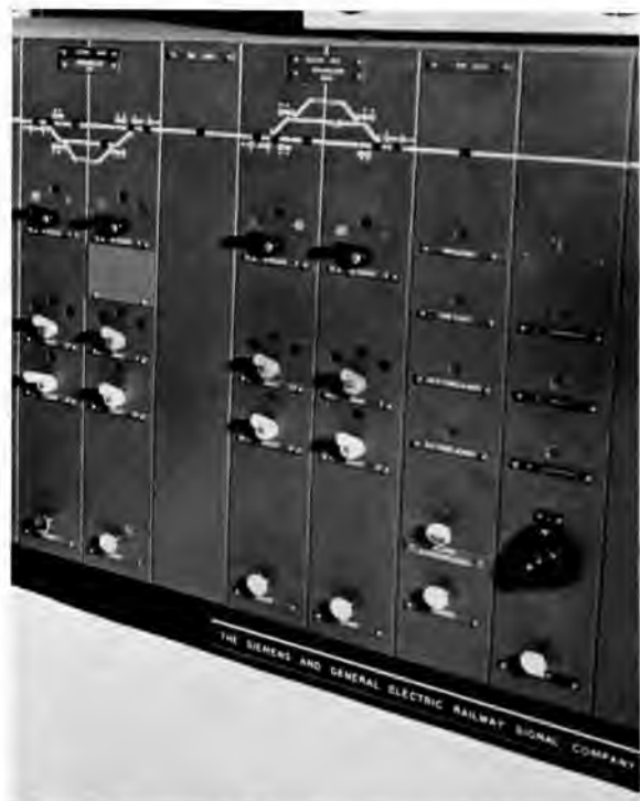
Fig. 11.—Close up of part of control-machine operating panel at Bulawayo.
