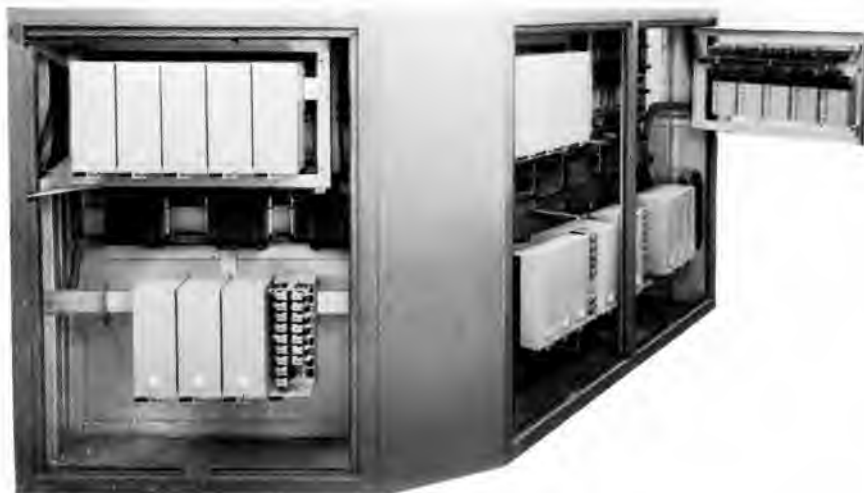
Fig. 12.—Rear view of control machine at Bulawayo.
