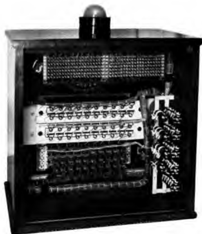
Fig. 4. Rear view of the Supervisor's control cabinet.
