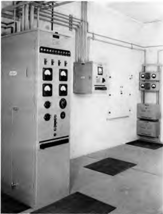
Fig. 9.—The control and remote terminal equipment at Bristol.
