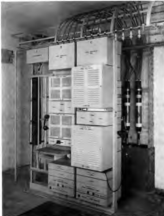
Fig. 3.—Line equipment on right hand rack. The power unit and supervisory equipment are mounted at the rear.
