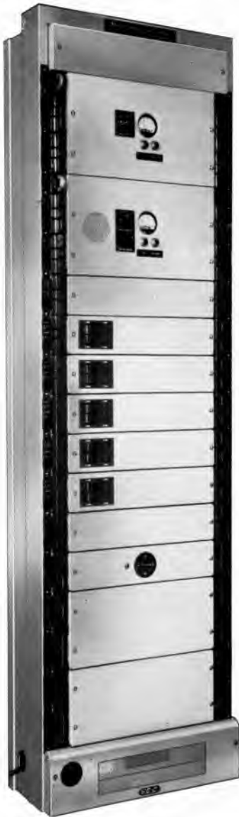
Fig. 1.—Five-circuit terminal rack.
