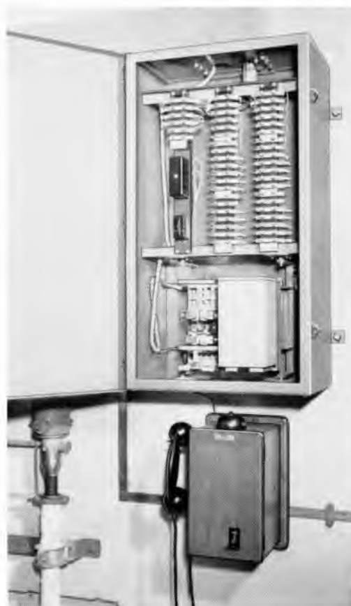
Fig. 14.—T.P. hut supervisory-control equipment.
